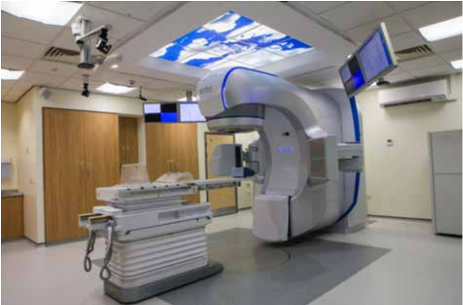
A photograph of a treatment unit
